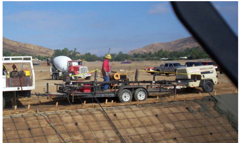
The Ditch Bank Rig mounted on a towable utility trailer, screeding a spillway
